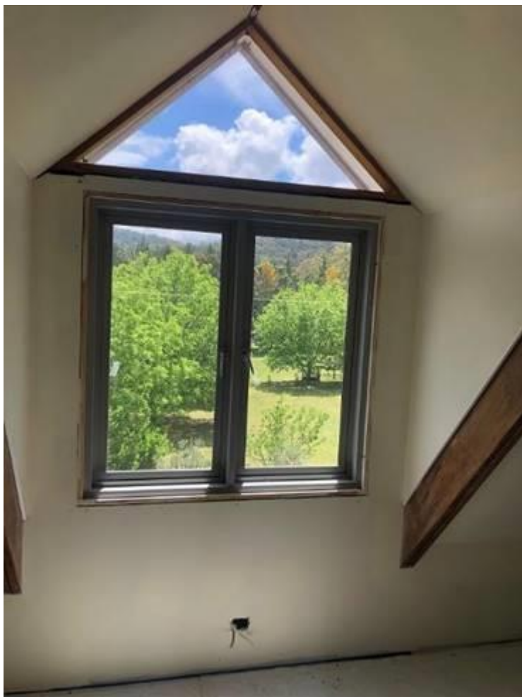
The first coat of paint! This is one of the upstairs accommodation rooms with beautiful views of the farm and surrounding hills. Below A spacious upstairs corridor.
